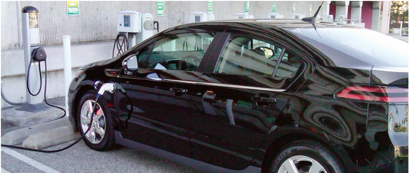
Figure 1. A Chevy Volt charges up with public Level 2 EVSE at Los Angeles International Airport. Photo from Coulomb Technologies
